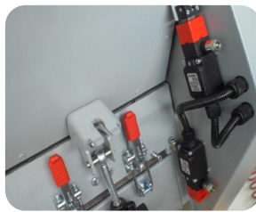
Two safety switches
