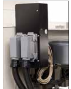
Quick change heater disconnects
